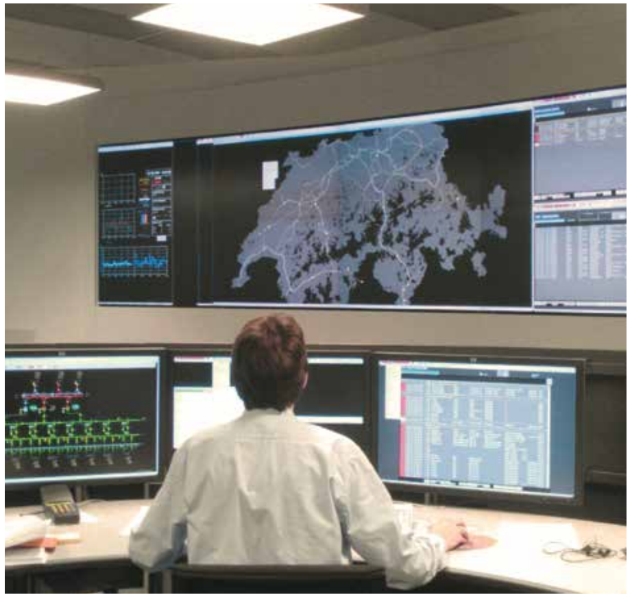
PSIcontrol control room at Swiss Federal Railways.
